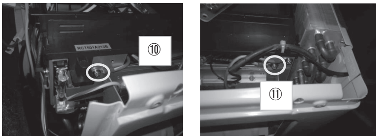
Fig.5 Earth cable of control box
